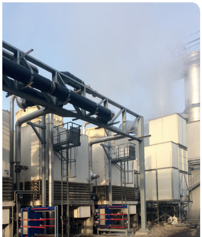
Existing cooling towers, which will, in the future, only be used as back-up if the district heating system cannot receive the surplus heat from the process at CP Kelco
